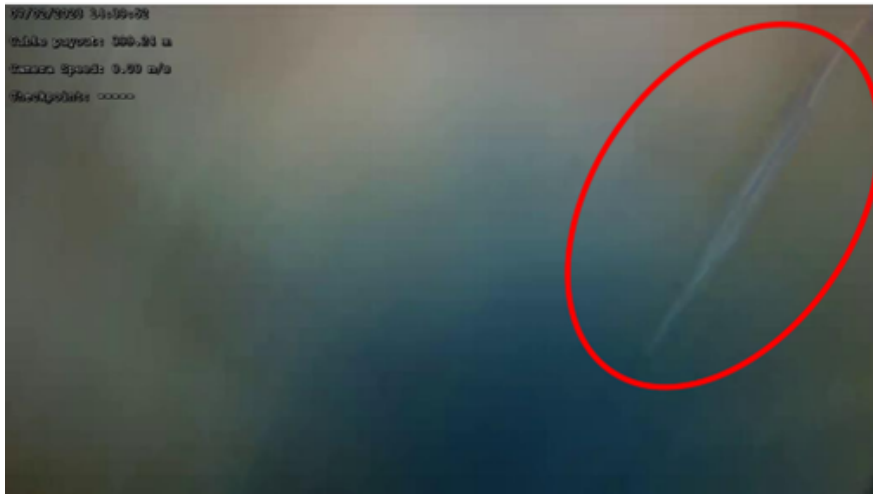
Longitudinal crack with leakage
